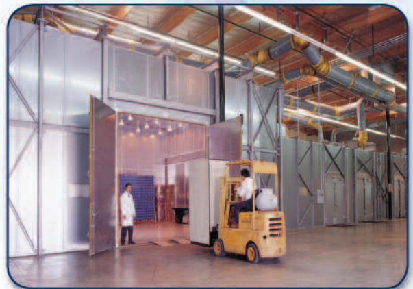
Shielded and Anechoic Chambers available at locations worldwide.
